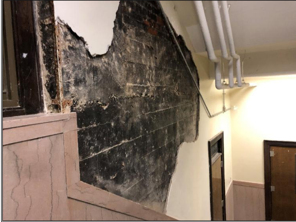
Photo 1: Damaged Plaster Wall
