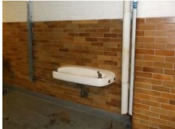
Typical Drinking Fountain
