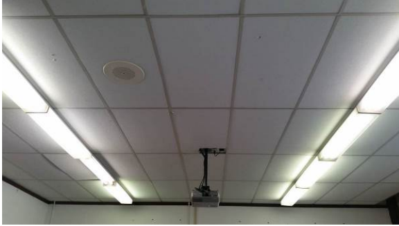
Typical Classroom Lighting
