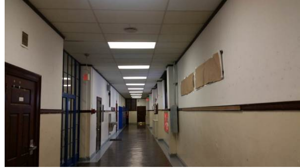
Typical Corridor Lighting
