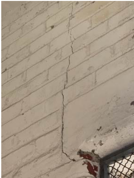
Cracking in Exterior Stairwell
