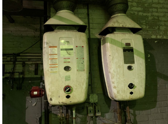
Hot water system
