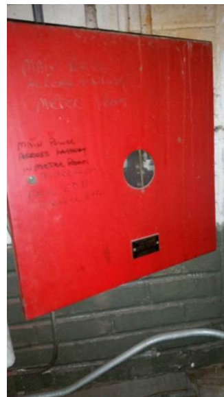
Fire Alarm Panel
