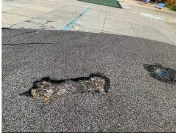
Failing Safety Surface
