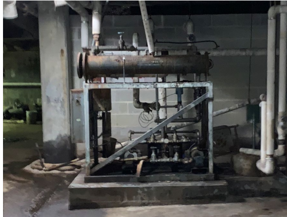
Fuel Delivery System
