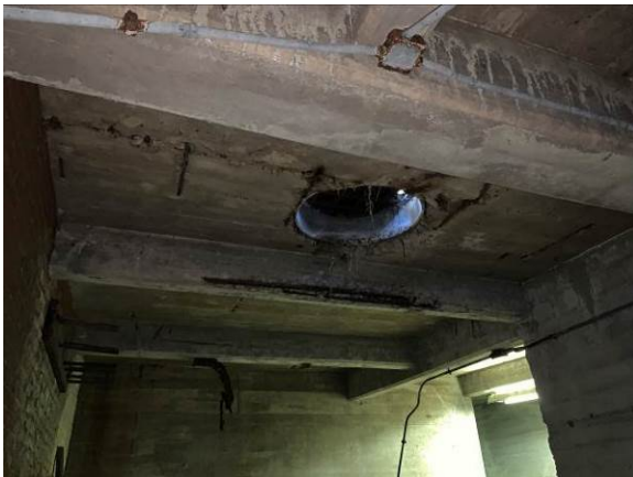
Fuel Storage Room
