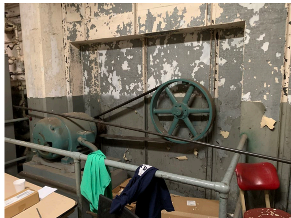
Building House Fan
