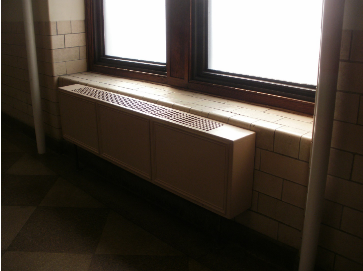
Photo No. 17 – Existing surface mounted low pressure steam radiator located in the corridor.
