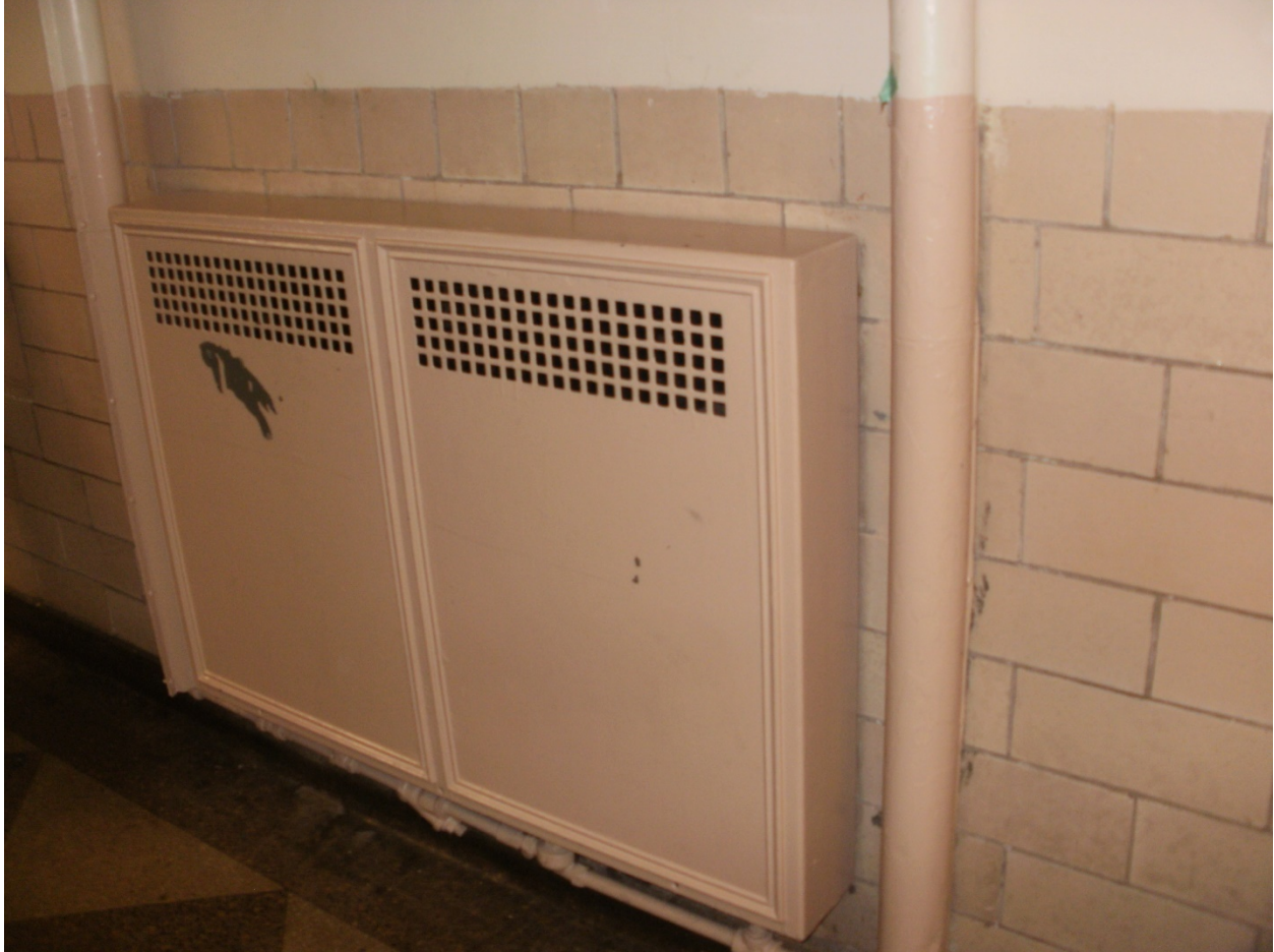
Photo No. 12 – A typical surface mounted low pressure Steam radiator located in the corridor area.
