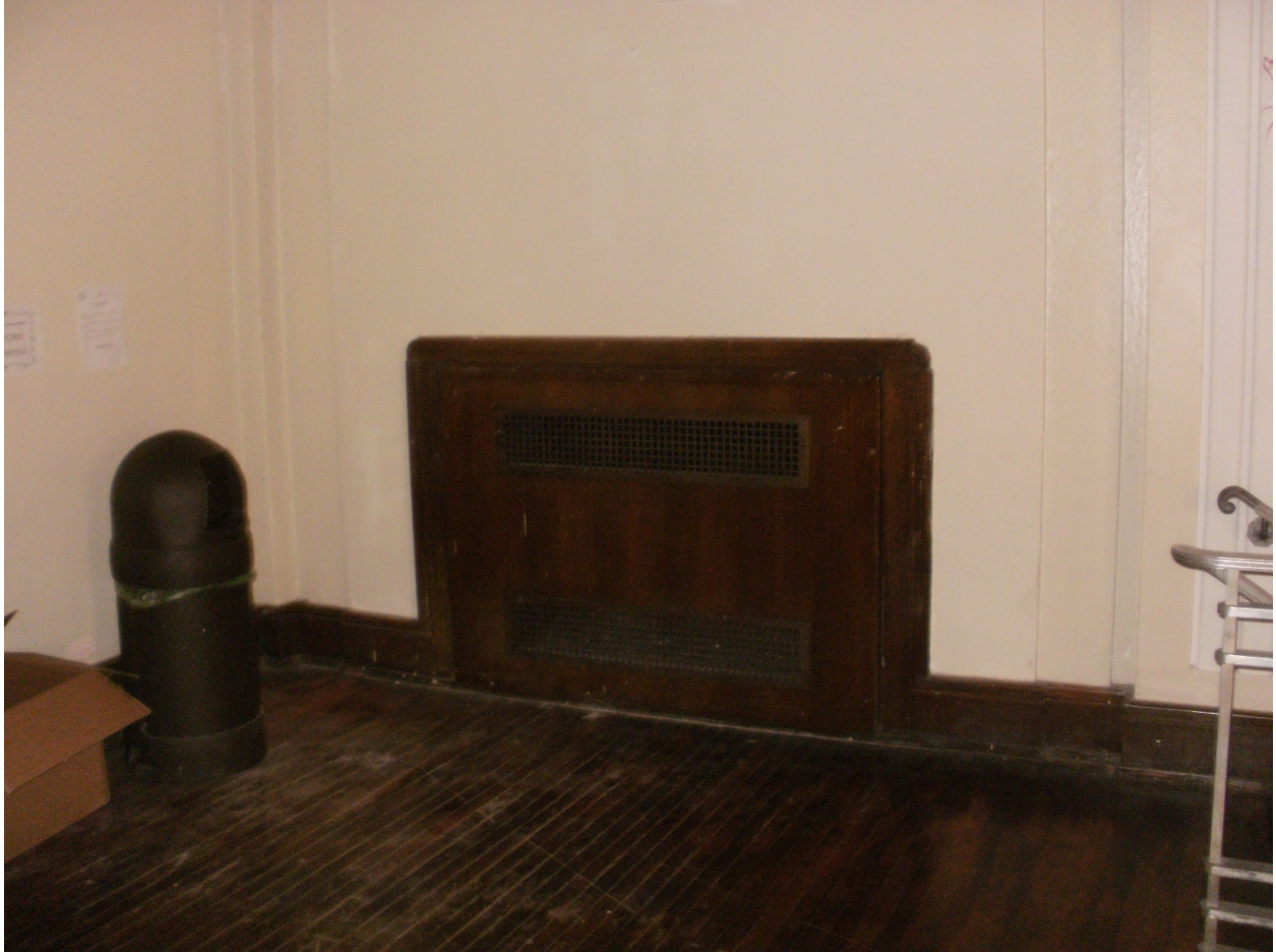
Photo No. 19 – Existing recessed wall mounted Low pressure steam radiator located behind the auditorium stage.
