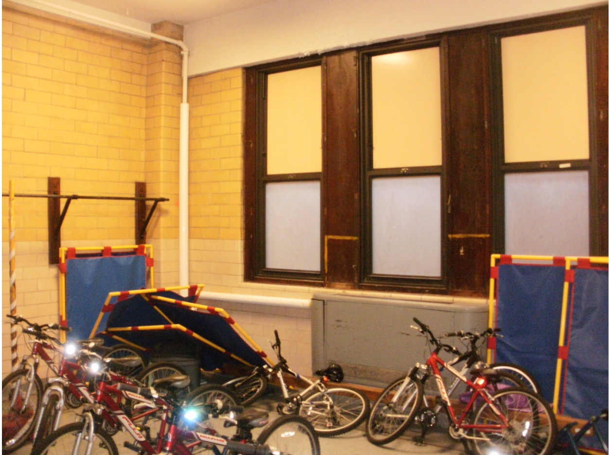
Photo No. 11 – An existing surface mounted low pressure steam radiator located in the gym common area.
