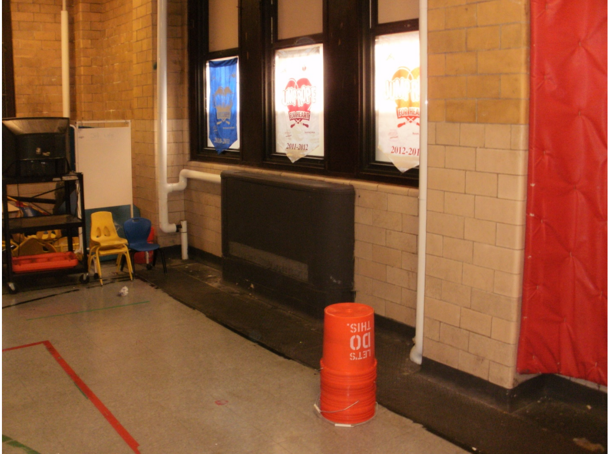
Photo No. 10 – A typical surface mounted low pressure steam radiator located in the cafeteria/gym areas.
