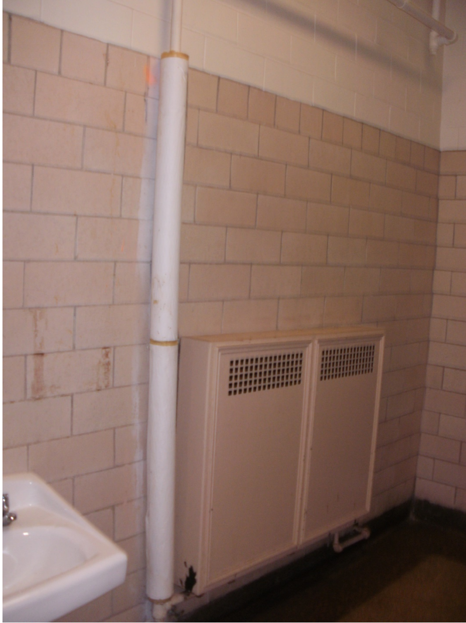
Photo No. 21 – Existing Bathroom Surface Wall Mounted Low Pressure Steam Radiators
