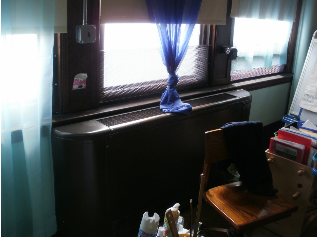
Photo No. 15 – A typical surface mounted low pressure Steam radiator located in the classroom
