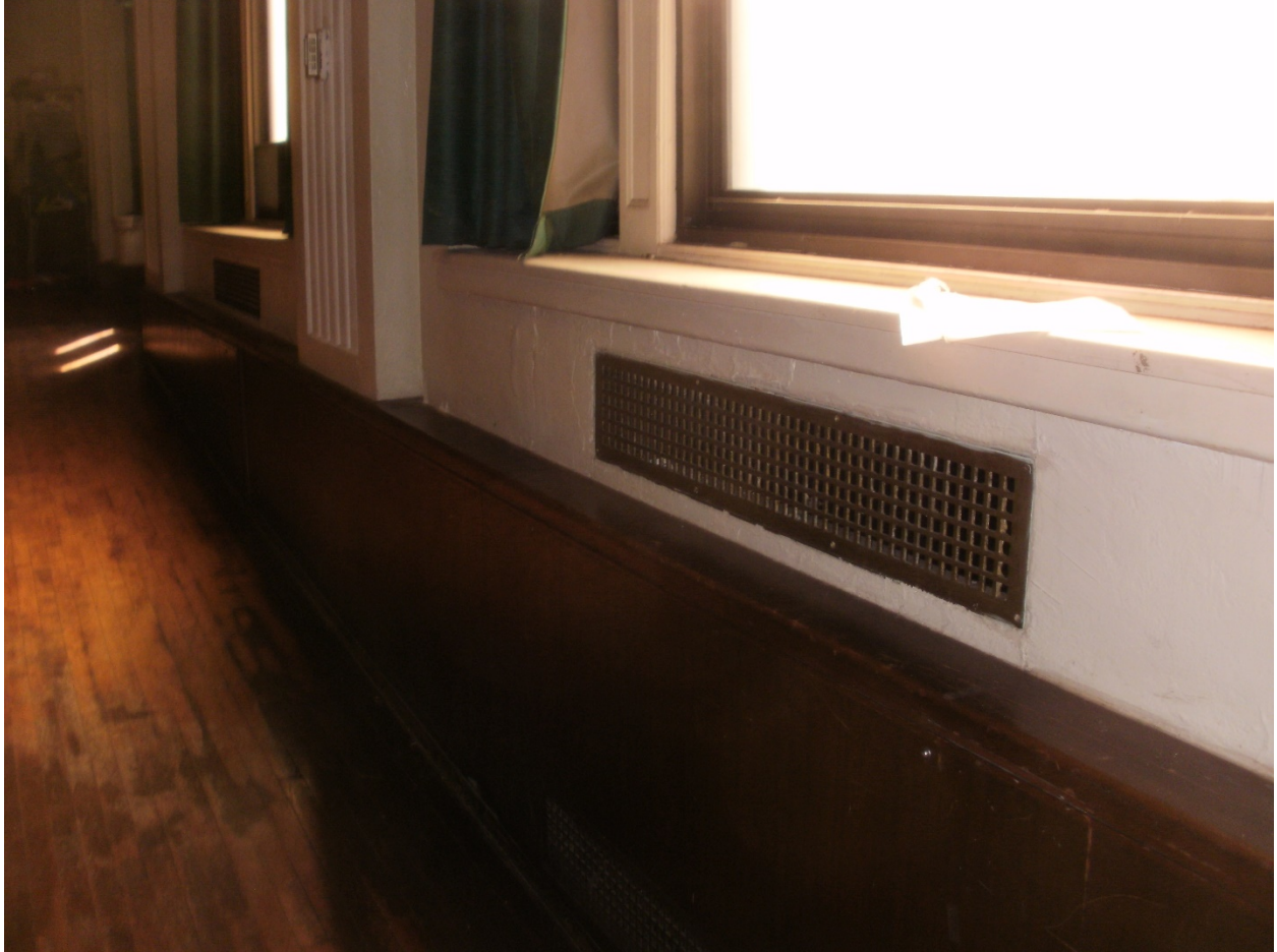
Photo No. 18 – Existing recessed low pressure steam Radiator located on the exterior wall of the auditorium
