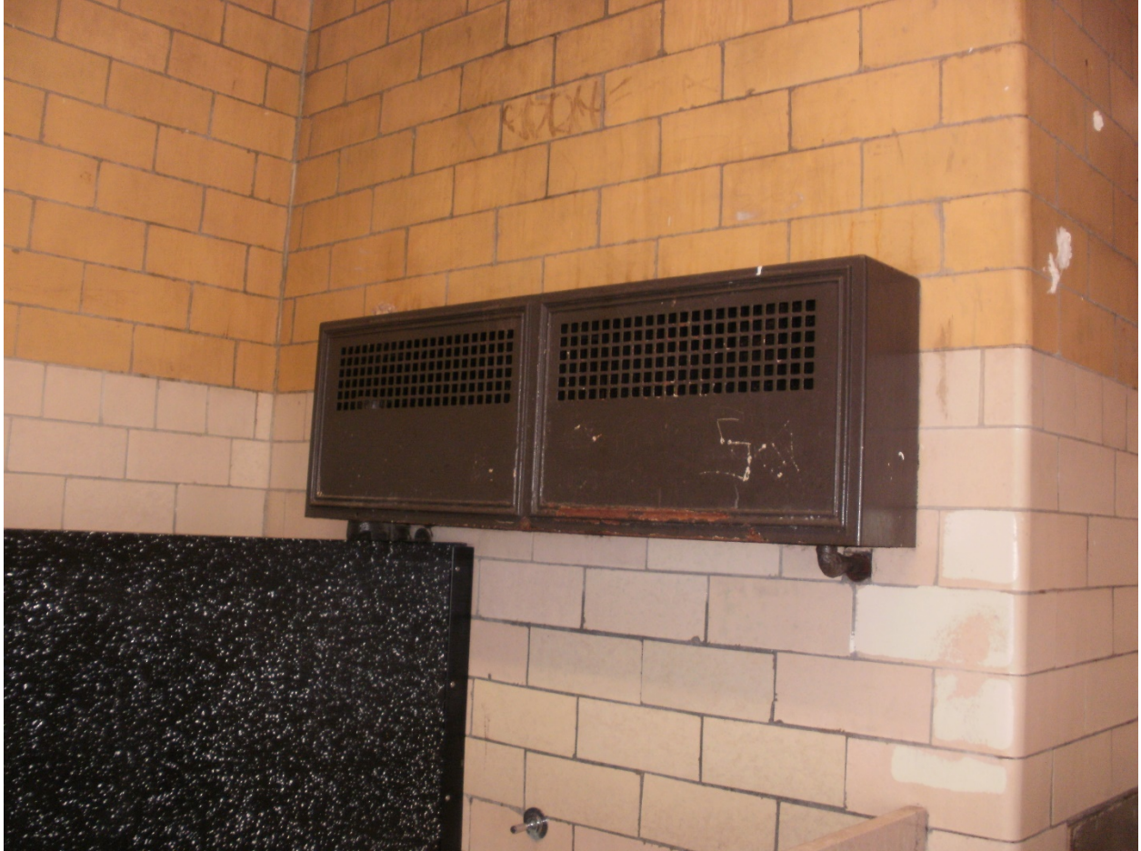
Photo No. 16 – An atypical elevated wall mounted low pressure steam radiator
