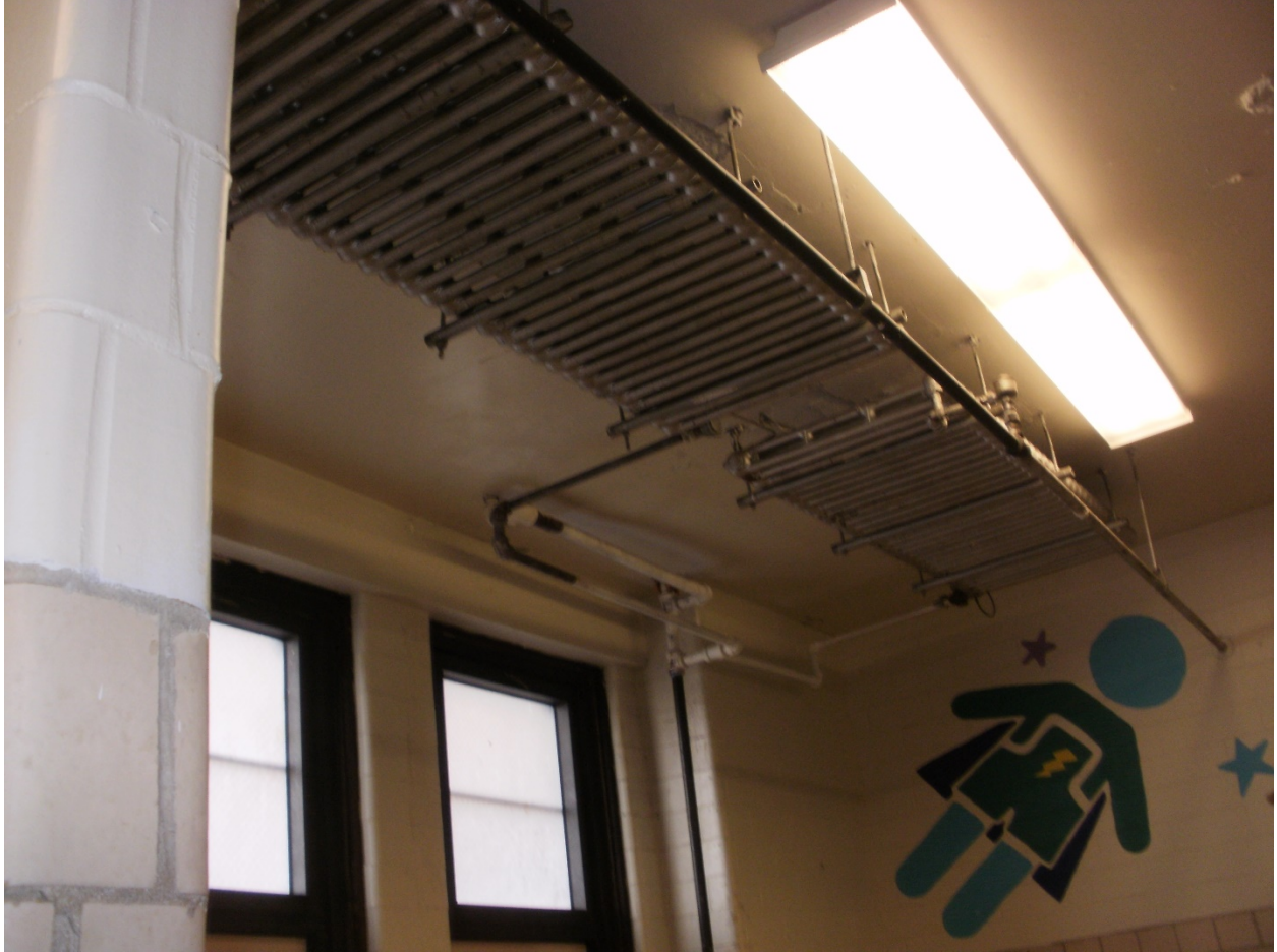
Photo No. 22 – Existing Cafeteria Ceiling Mounted Low Pressure Steam Radiators
