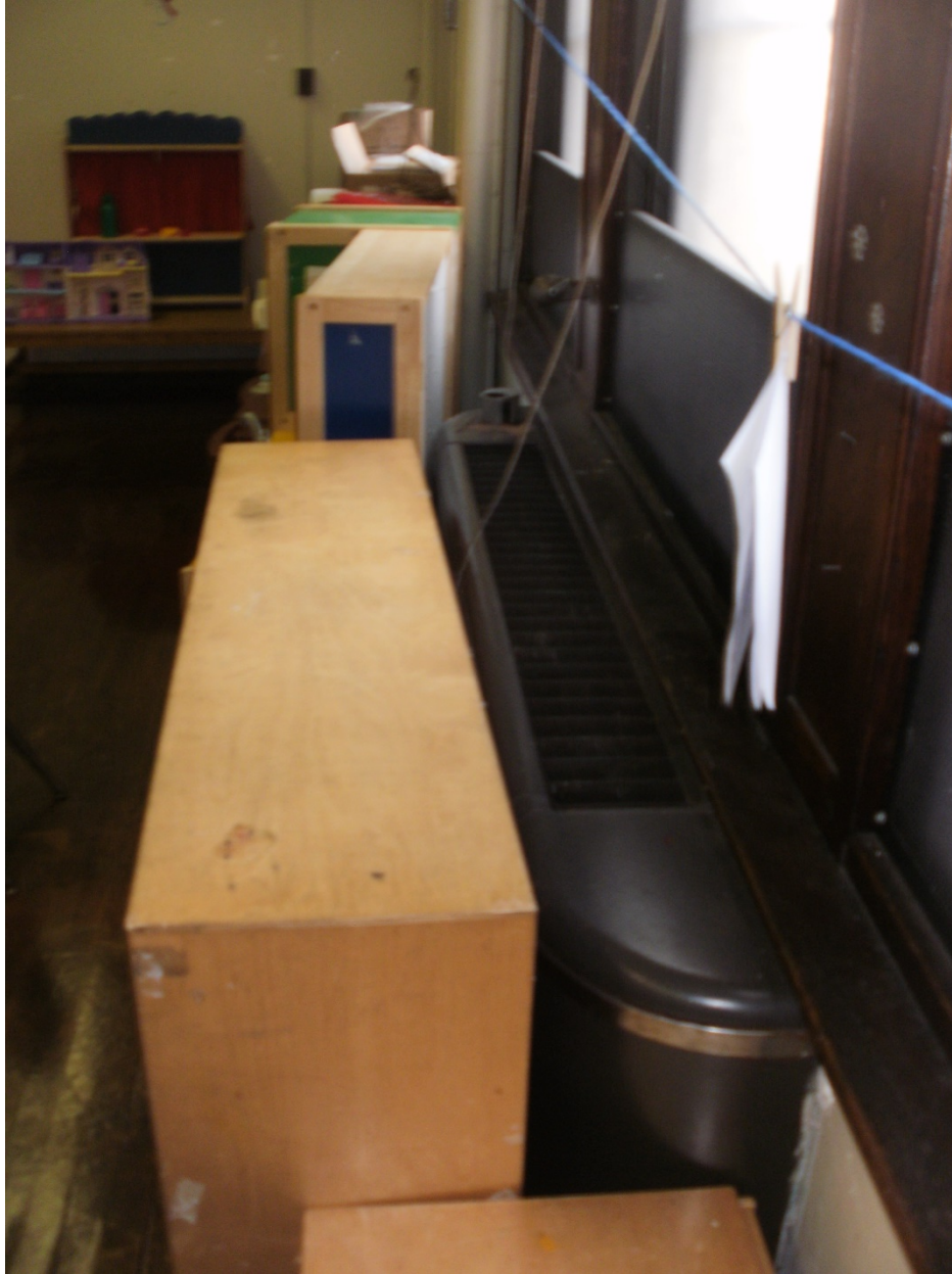
Photo No. 13 – A typical surface mounted low pressure Steam radiator located in the classroom
