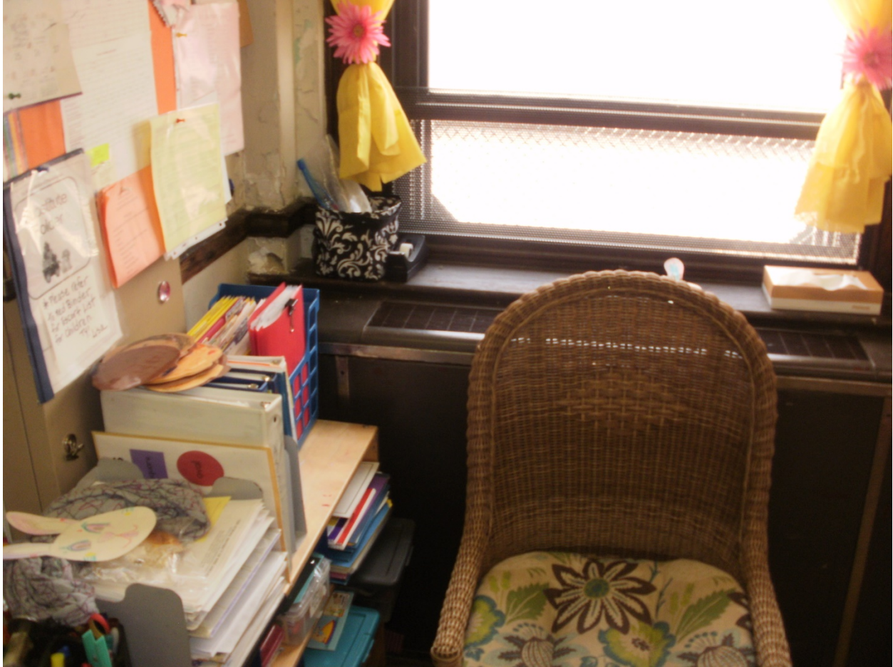
Photo No. 14 – A typical low pressure steam surface mounted corner radiator located in a classroom.
