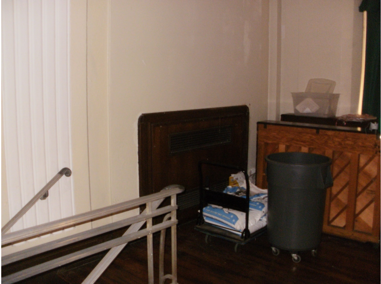
Photo No. 20 – Existing Low Pressure recessed Wall Mounted Steam Radiators Located Behind the Auditorium Stage Area
